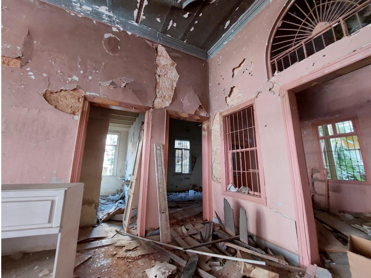
Figure 31: An unrepaired severely damaged house. October 2021. Photo: Abir Zaatari.
