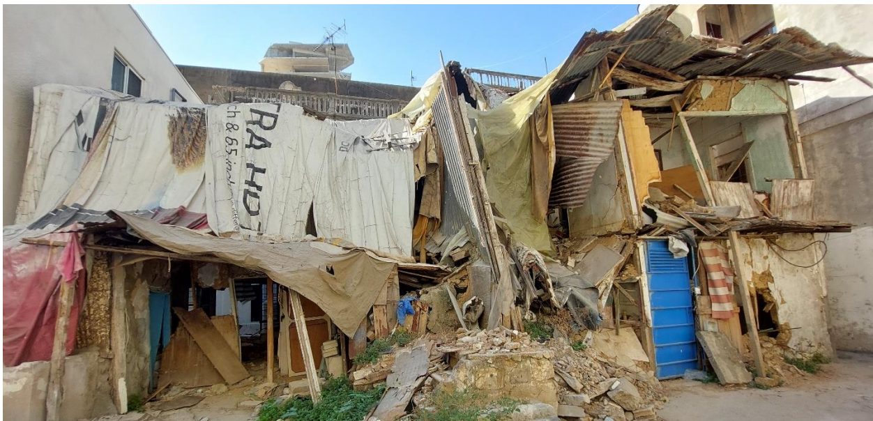
Figure 32: A fragile structure severely damaged after the blast. September 2021. Photo: Abir Zaatari.
