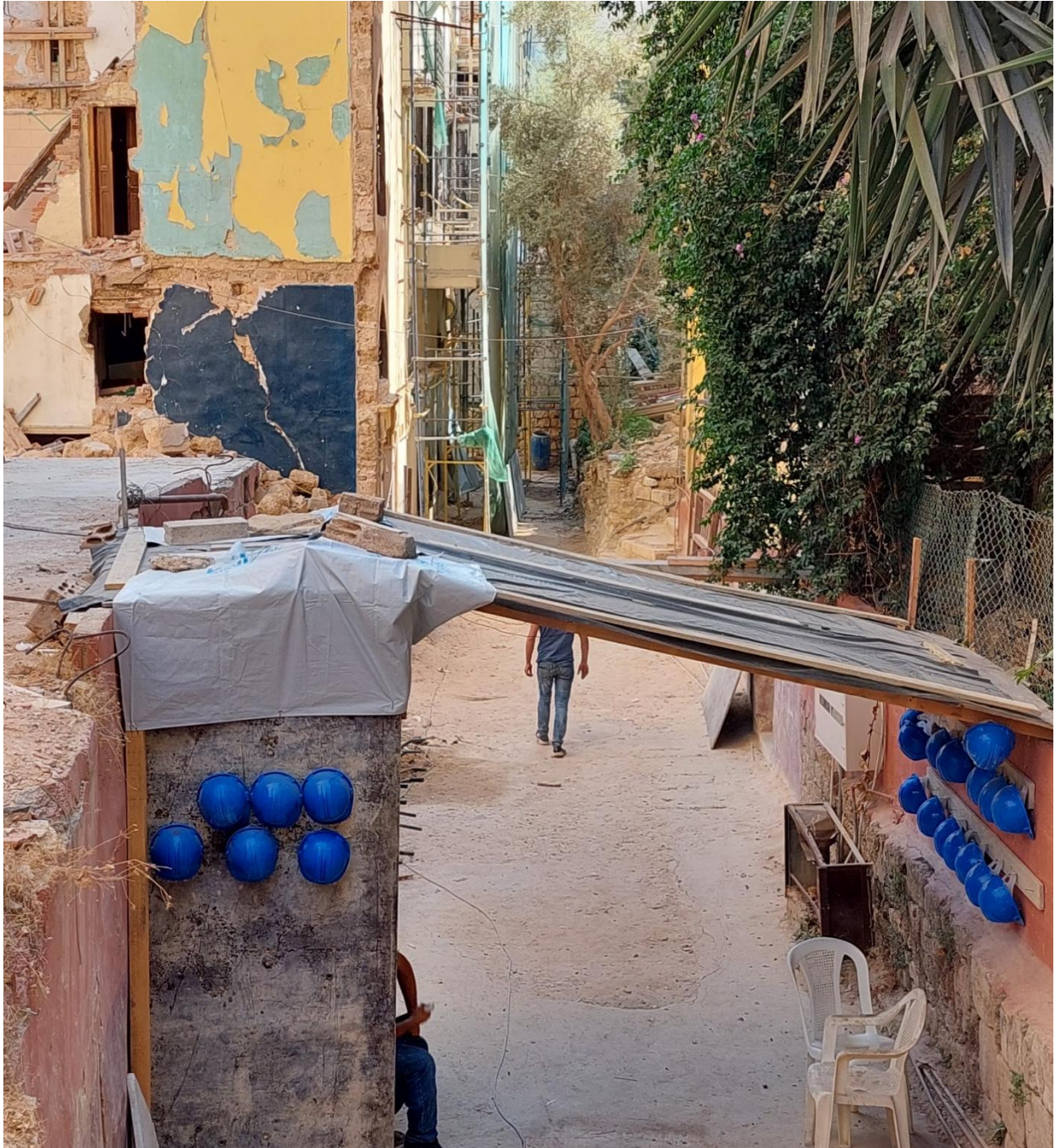
Figure 24: Ongoing repair works after almost one year and a half since the blast, October 2021. Photo: Abir Zaatari.
