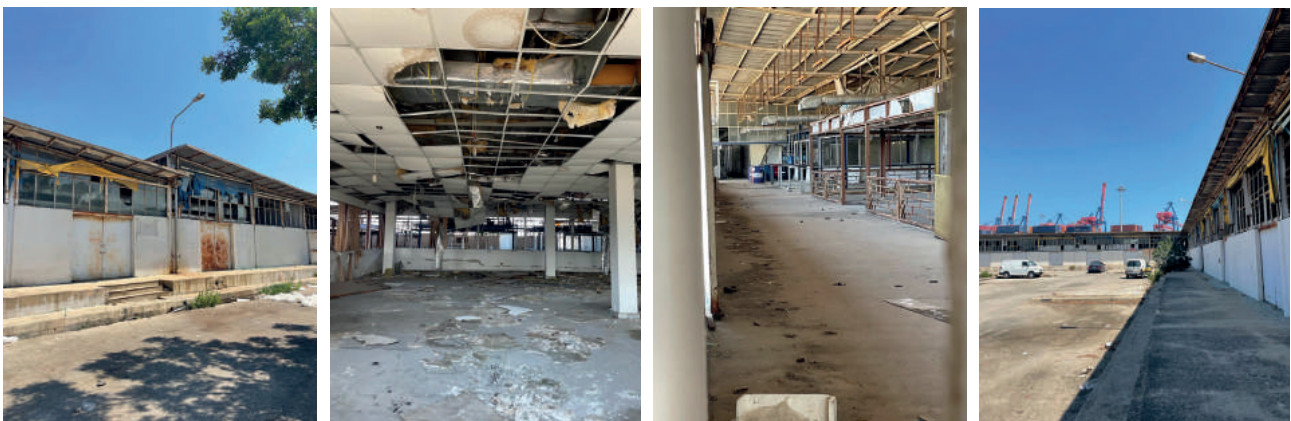
Figure 16. The abandoned public market near the fish market. Source: Cristina Gosen, 2022.
