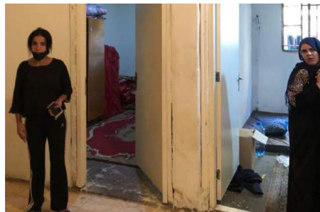
Figure 11: The interior of a residential building showing the poor installation of a door after the port blast. Source: Abir Cheaitli, 2021.
