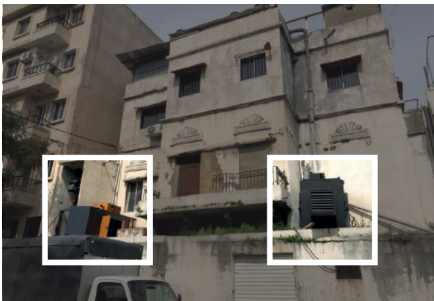
Figure 29c. Two private generators that are located at the top floor of a building because of the lack of space on the ground level. Source: Abir Cheaitli, 2021.
