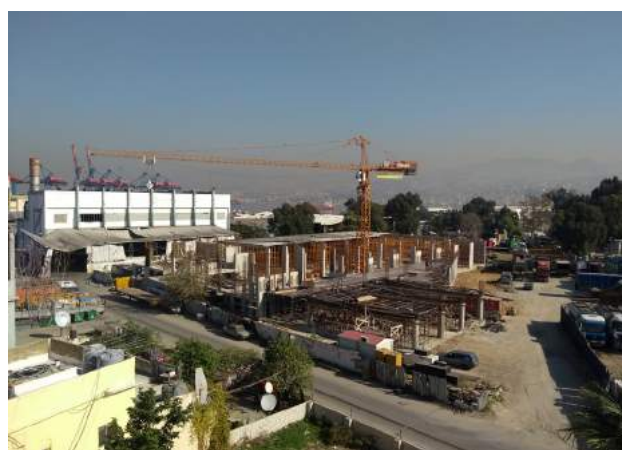
Figure 70. A building with a porch that is under construction in the Industrial Zone. Source: Ali Ghaddar, 2021.
