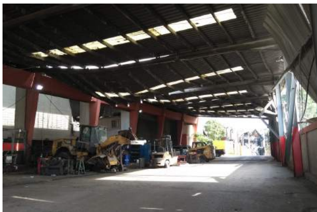
Figure 47. An interior view of the waste management facility after the port blast. Source: Ali Ghaddar, 2021.
