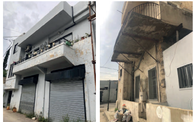
Figure 7: The images above show the exterior conditions of residential buildings. Source: Abir Cheaitli, 2021.
