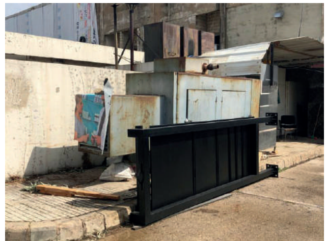
Figure 29d. Private generators providing electricity to warehouses that are used to store medicine for the governmental hospital. Source: Abir Cheaitli, 2021.
