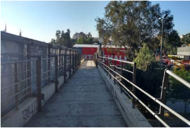
Figure 7. The physical quality of the pedestrian overpass from Karantina to Mar Mikhael: the structure of the overpass does not include a shaded roof and the handrail is damaged. Source: Ali Ghaddar, 2021.
