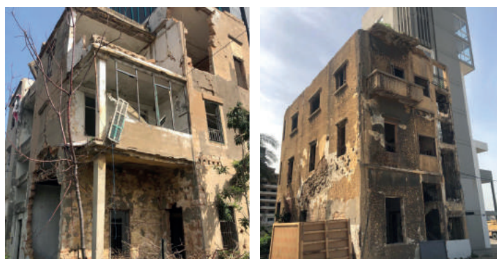
Figure 3. The physical condition of abandoned buildings, Karantina. Source: Abir Cheaitli, 2021.
