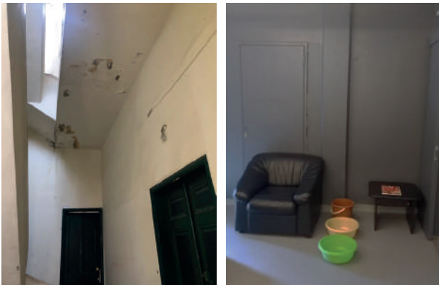
Figure 6: The images above were taken from inside the residential buildings, showing traces of severe mold, humidity, and dampness. Source: Abir Cheaitli, 2021.
