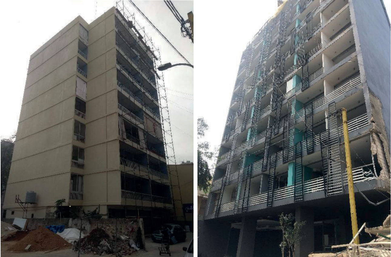
Figure 5. Housing typologies in Al-Saydeh I sub-neighborhood from the 1980s onwards. Source: Abir Cheaitli, 2021.
