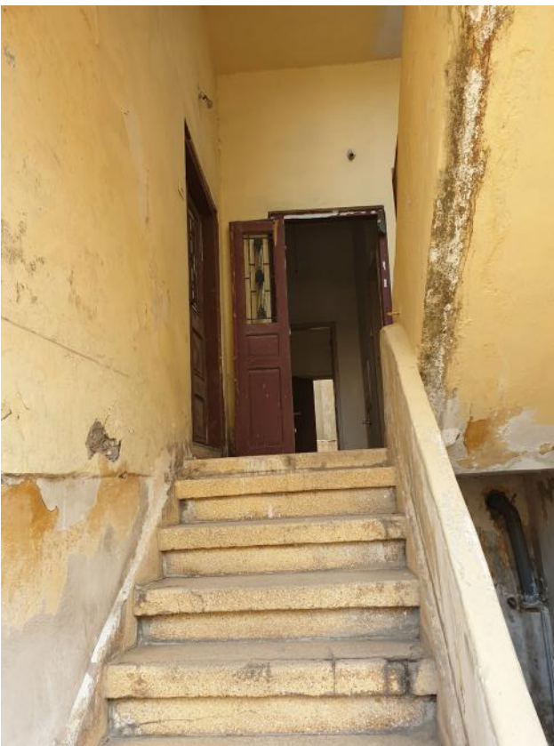
Figure 37. Poor quality of a residential building in Karantina. Source: Batoul Yassine, 2021.
