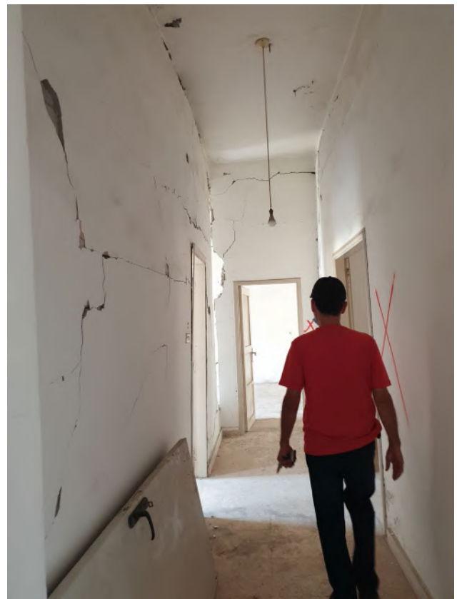
Figure 38. A structurally damaged residential apartment in AL-Khodor sub-neighborhood by the port blast. Source: Batoul Yassine, 2021.
