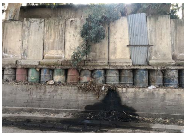
Figure 22. Inaccessible concrete walls on the sidewalks in the industrial area. Source: Abir Cheaitli, 2021.
