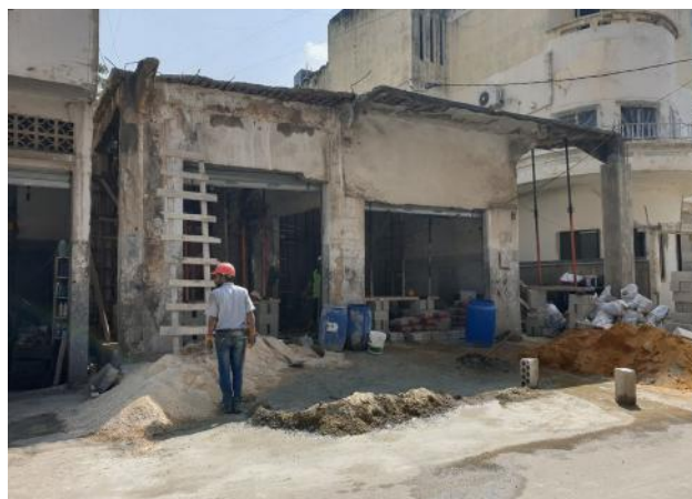
Figure 29. Another car garage being renovated after the port explosion. Source: Batoul Yassine, 2020.
