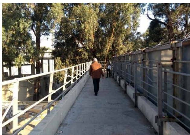
Figure 13. The pedestrian bridge that runs over the Charles Helou Highway. Source: Abir, Cheaitli, 2021.
