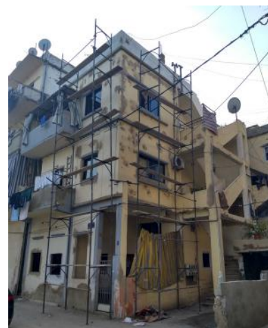
Figure 14. Renovation of a residential building in process after the port blast. Source: Abir Cheaitli, 2021.
