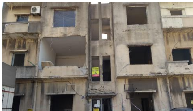
Figure 13. Deteriorating residential building. Source: Abir Cheaitli, 2021.
