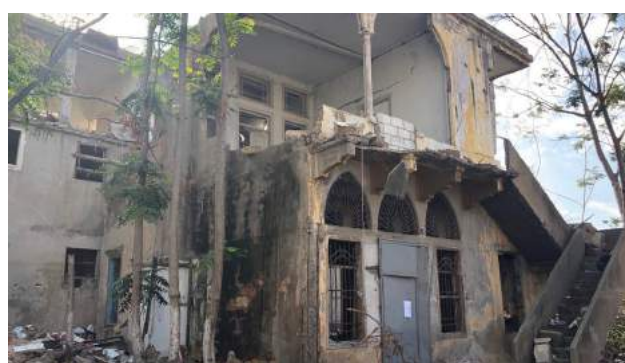
Figure 11. Abandoned and deteriorated buildings. Source: Abir Cheaitli, 2020
