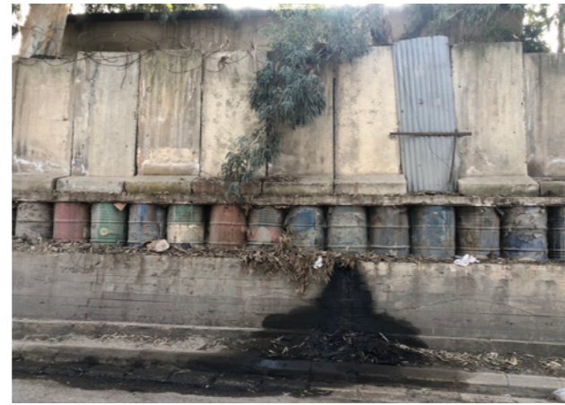
Figure 22. Inaccessible concrete walls on the sidewalks in the industrial area. Source: Abir Cheaitli, 2021.
