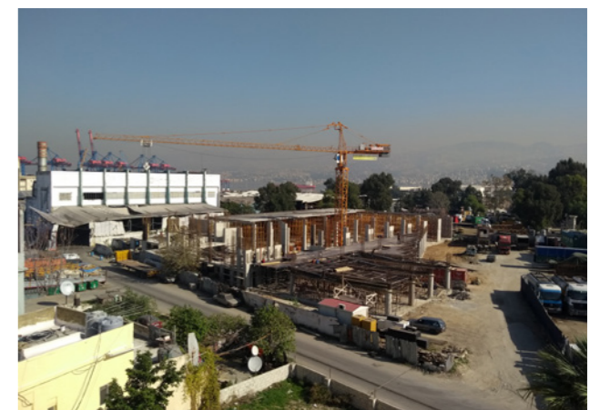
Figure 70. A building with a porch that is under construction in the Industrial Zone. Source: Ali Ghaddar, 2021.
