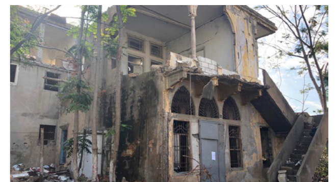
Figure 11. Abandoned and deteriorated buildings. Source: Abir Cheaitli, 2020
