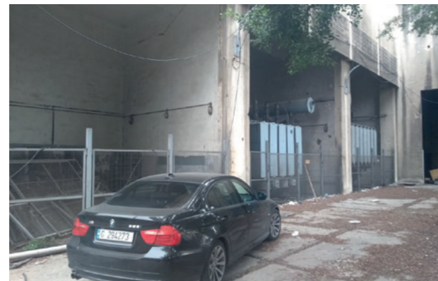
Figure 27. The EDL building in Karantina. Source: Ali Ghaddar, 2021.
