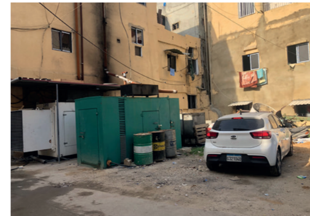
Figure 29b. Generators that serve residential houses. Source: Abir Cheaitli, 2021.
