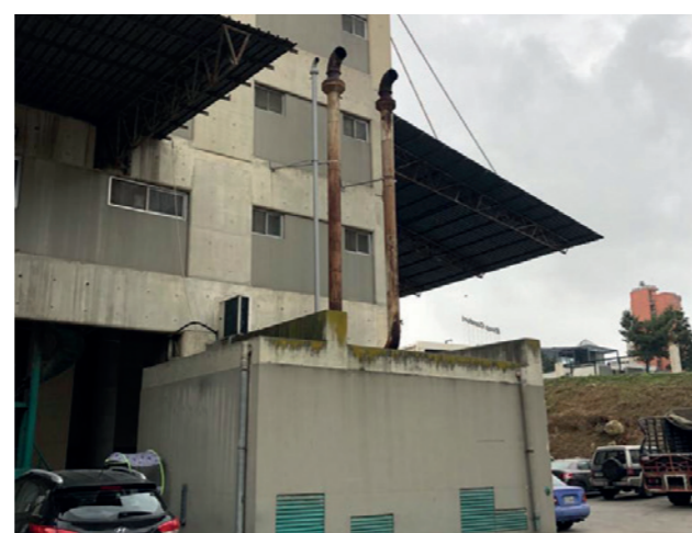
Figure 29a: The electrical generator of the Bakalian flourmills. Source: Abir Cheaitli, 2021.
