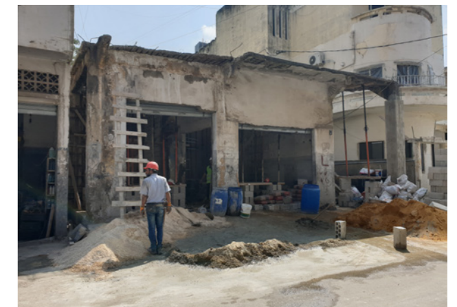
Figure 29. Another car garage being renovated after the port explosion. Source: Batoul Yassine, 2020.
