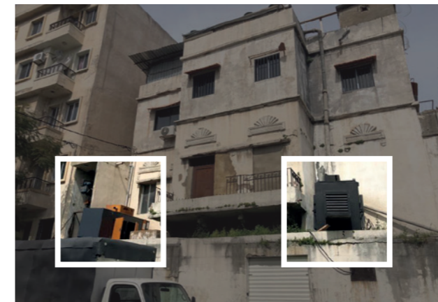
Figure 29c. Two private generators that are located at the top floor of a building because of the lack of space on the ground level. Source: Abir Cheaitli, 2021.
