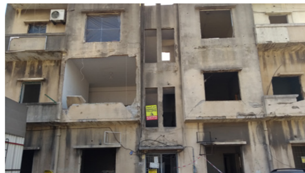
Figure 13. Deteriorating residential building. Source: Abir Cheaitli, 2021.
