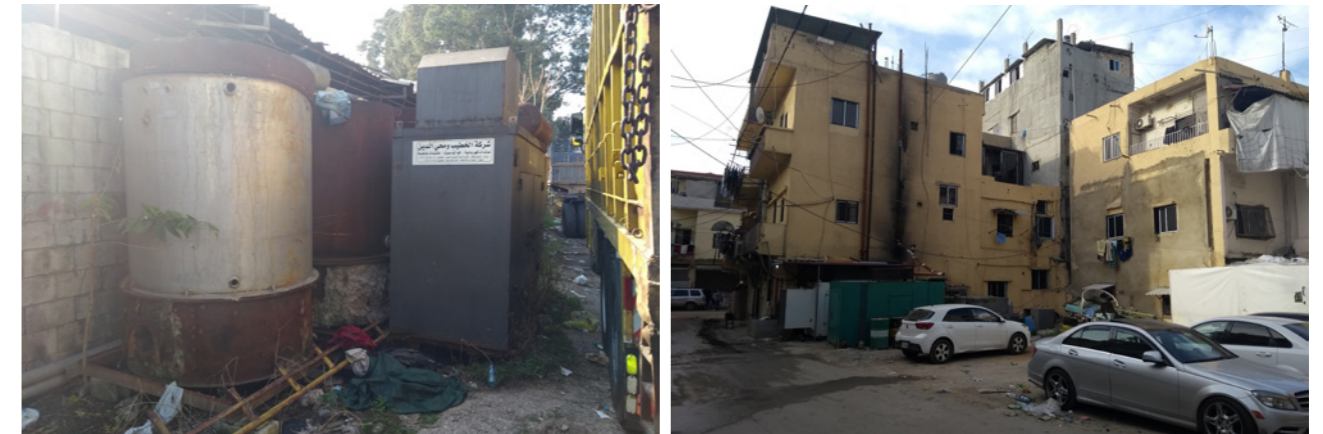
Figure 49. Private generators placed near residential buildings. Source: Abir Cheaitli, 2021.
