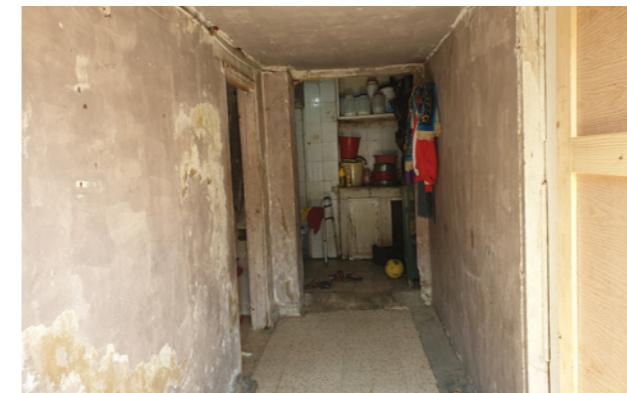
Figure 10. The indoor quality of a residential house in Al-Khodor sub-neighborhood. Source: Batoul Yassine, 2020.
