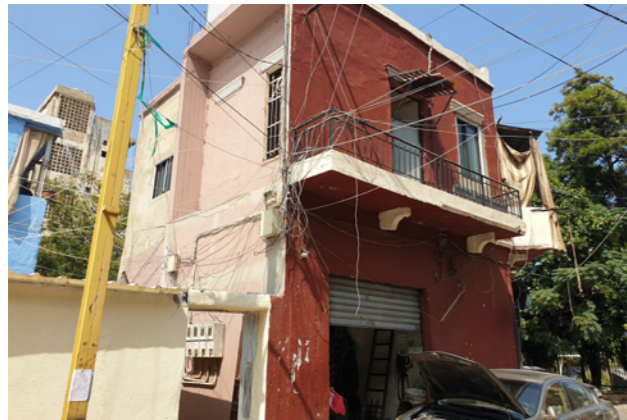
Figure 39. Informal electrical hook-ups on an electrical pole. Source: Batoul Yassine, 2021.
