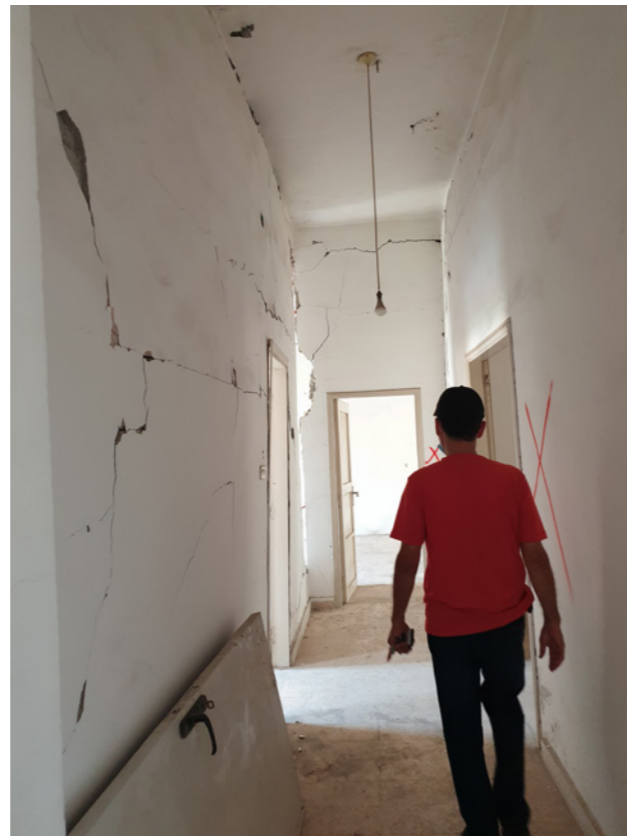
Figure 38. A structurally damaged residential apartment in AL-Khodor sub-neighborhood by the port blast. Source: Batoul Yassine, 2021.
