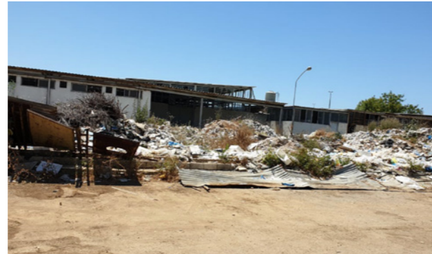
Figure 5. The dilapidated condition of the current slaughterhouse in Karantina. Source: Abir Cheaitli, 2021.
