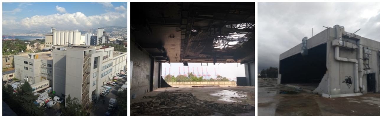
Figure 95. The destroyed roof of the Food Wholesale building. Source: Ali Ghaddar, 2021.
