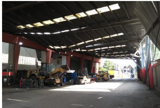
Figure 47. An interior view of the waste management facility after the port blast. Source: Ali Ghaddar, 2021.
