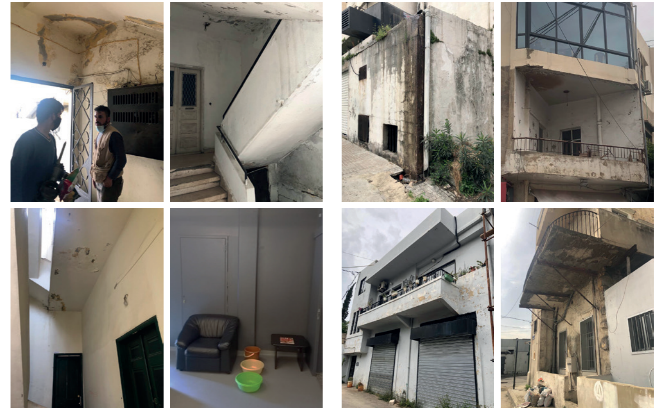
Figure 6: The images above were taken from inside the residential buildings, showing traces of severe mold, humidity, and dampness. Source: Abir Cheaitli, 2021.
