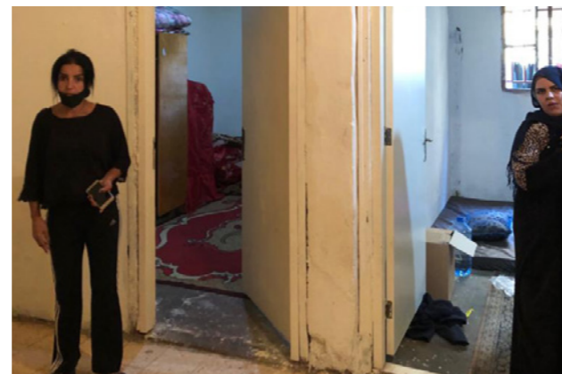
Figure 11: The interior of a residential building showing the poor installation of a door after the port blast. Source: Abir Cheaitli, 2021.
