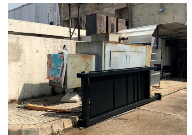
Figure 29d. Private generators providing electricity to warehouses that are used to store medicine for the governmental hospital. Source: Abir Cheaitli, 2021.
